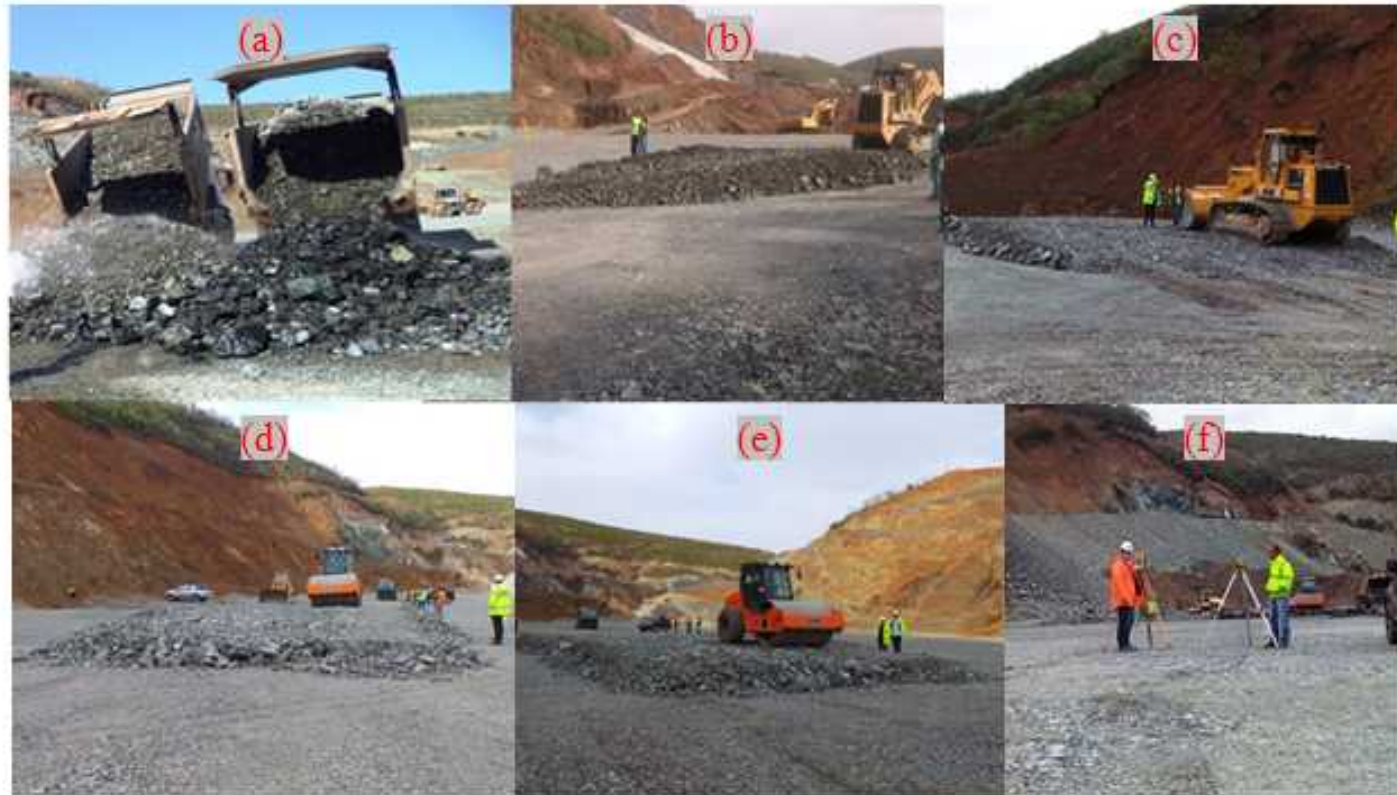
Figure 3 (a) Transporting the rockfill material from the quarry to the trial embankment area, (b) and (c) Preparing the trial embankment layer of 65,00 and 85,00 cm respectively, (d) and (e) 4, 6 and 8 roller passing per each respective layer, (f) Recording settlement for each point via topographic measurements.
